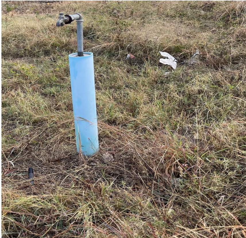
Picture 5.1: A dilapidated communal water tap
